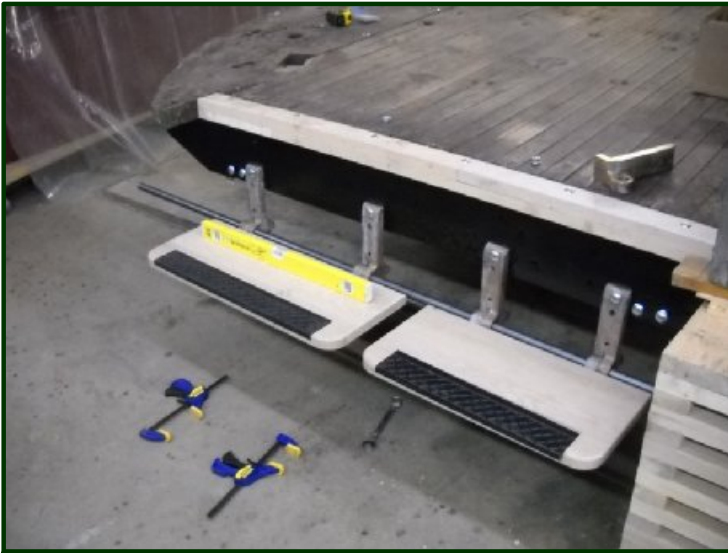
Probably the most complicated system on Winona No. 10, not counting the electrical components, will be the step operating mechanisms. Here the steps are just being test fitted to get an idea what they'll look like. This is not the step's final configuration.
