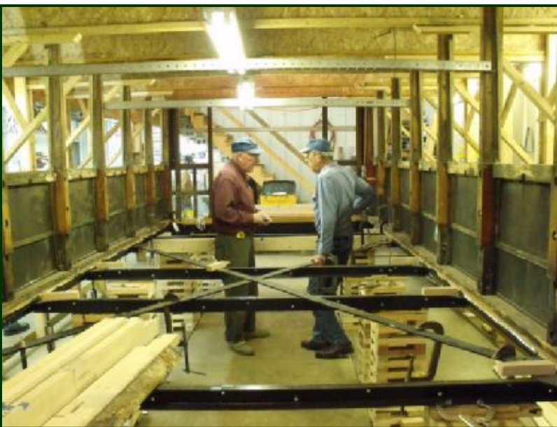
(Left) Here's Ken Albrecht (left) talking about the wood pieces of Winona No. 10's sub-structure with new volunteer Scott Ingram . Pieces of the wood can be seen in the lower left corner of the photo.
