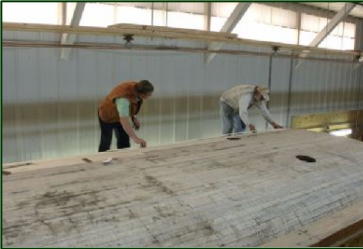
Many of Winona 10's roof board were good, but some others were in need of replacement. Here we see Jim Peschong (left) and Steve Mages checking the fit of one of the replacement wood roof pieces.
